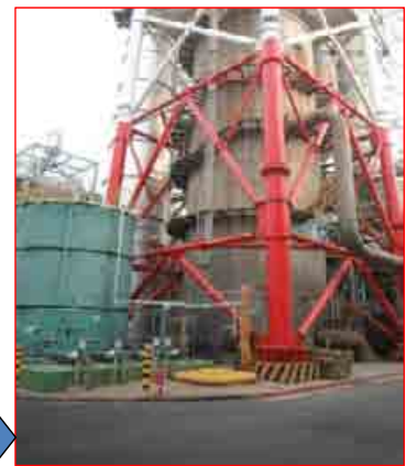
濕式洗滌塔(Wet Scrubber) 煙道氣排煙脫硫設備(FGD)
