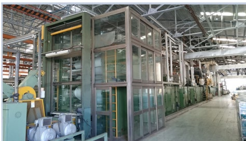
Enclosed negative pressure containment for the coating area of a polyurethane synthetic leather plant
