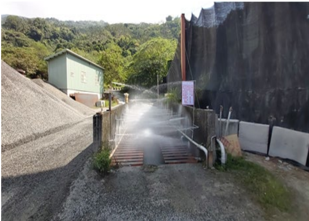
Bump-type car wash station
