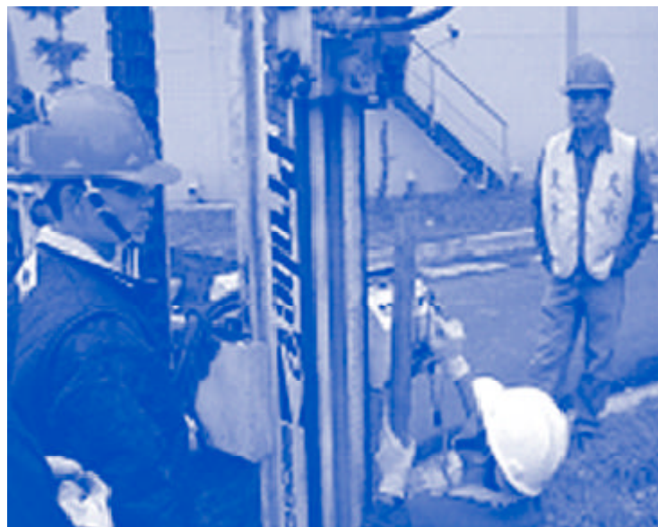
Drilling a temporary monitoring well during pollution investigation of petrochemical storage site.
